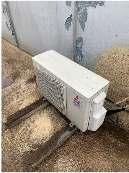
Existing Heat Pump
