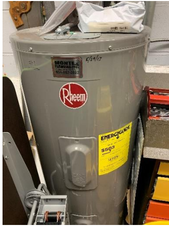
Existing Electric Domestic Water Heater
