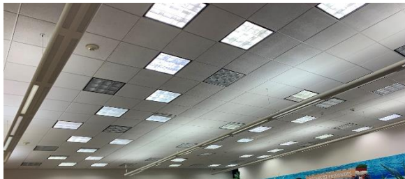
Existing Light Fixtures in Library
