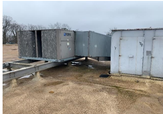
Existing Rooftop Unit – RTU-2
