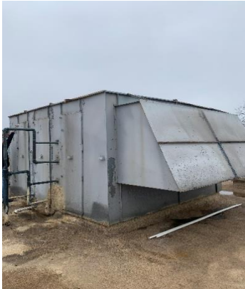
Existing Rooftop Units – RTU-1
